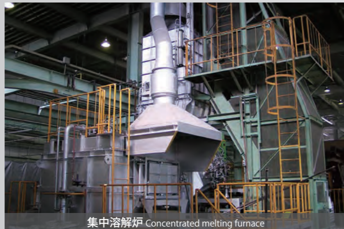
集中溶解炉 Concentrated melting furnace
